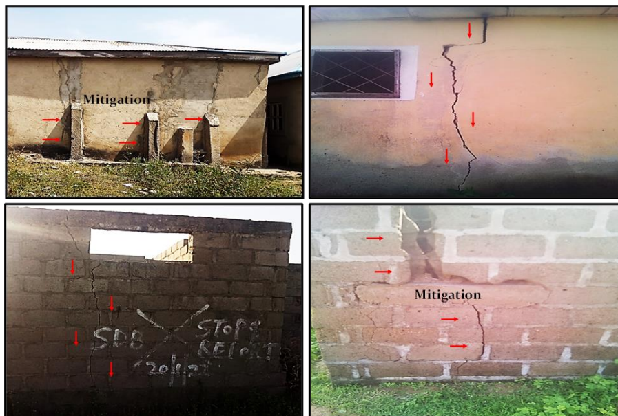
Figure 1: Mitigation measures on cracked building
