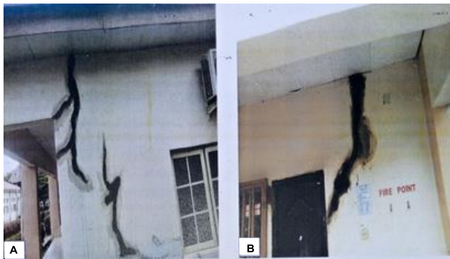
Plate 2: Cracks on the PG Economics Lab
