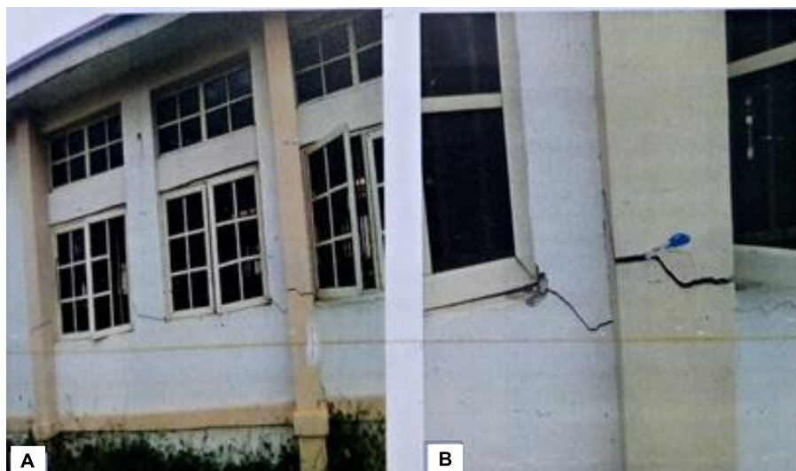
Plate 3: Cracks on the LLR4 Block
