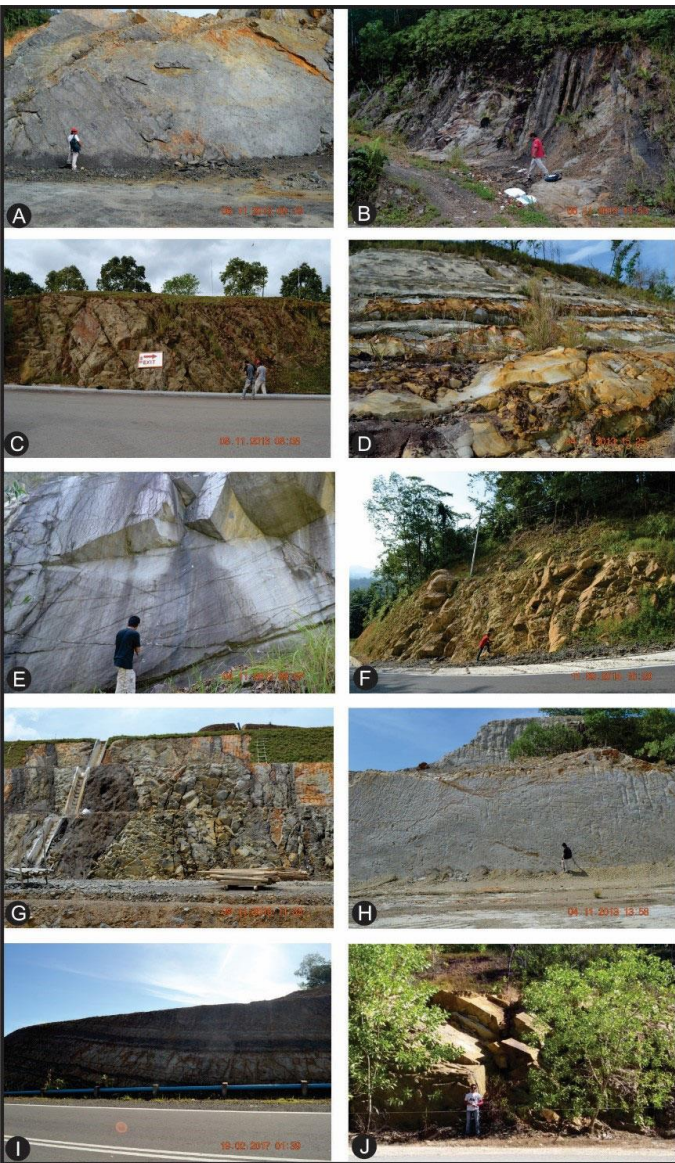
Figure 1: The selected slopes. Note: A- slope 1; B- slope 2; C- slope 3; D- slope 4; E- slope 5; F- slope 6; G- slope 7; H- slope 8; I- slope 9; J- slope 10.
